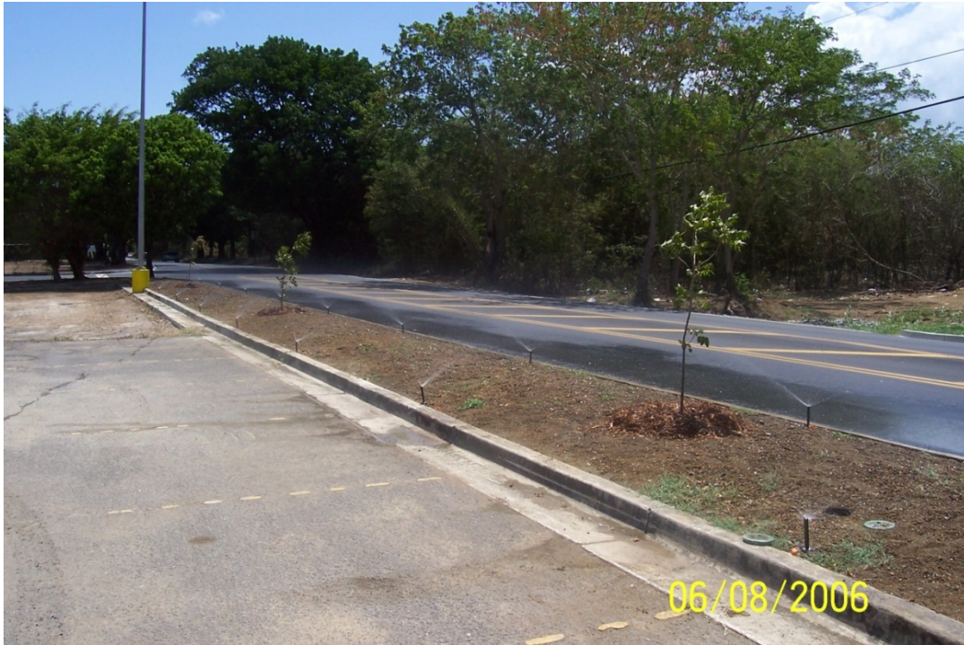
Queen Mary Highway, Sprinkler System, Station: 16+00 Rt.
