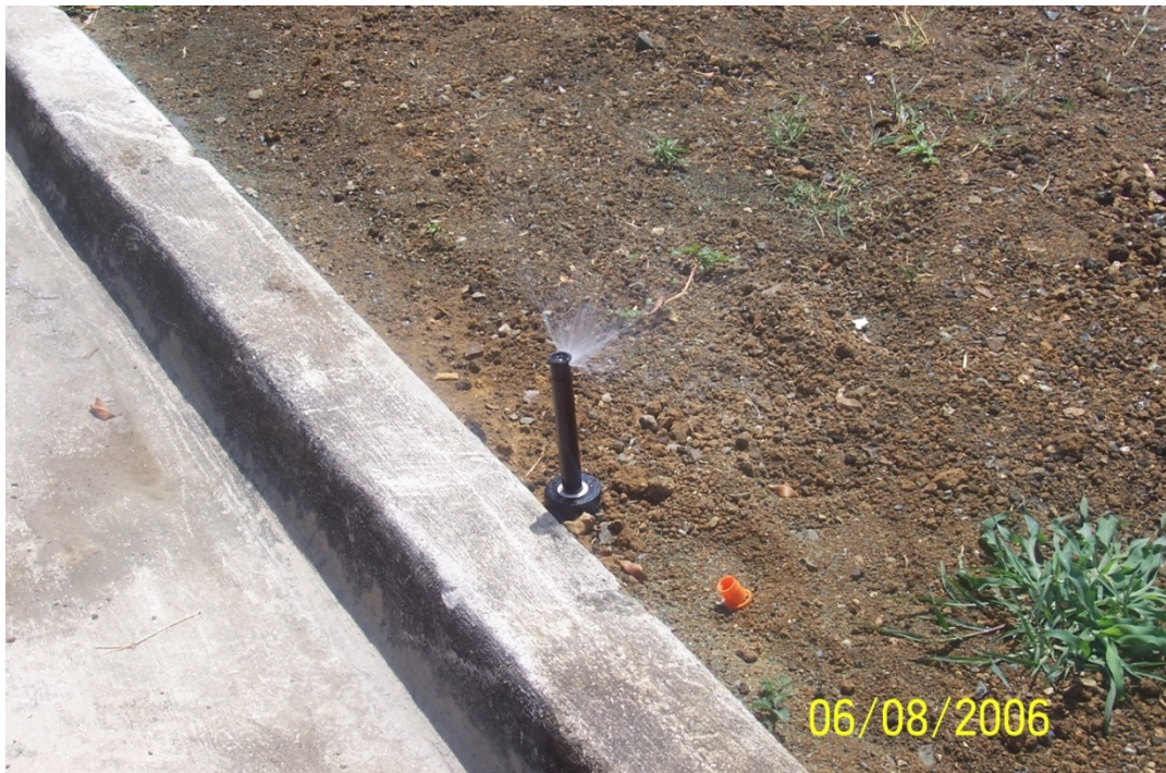
Queen Mary Highway, Sprinkler System, (Pop-up Spray Head) Station: 17+50 Rt.
