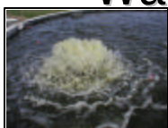
Aeration 3 vertical lift pumps
