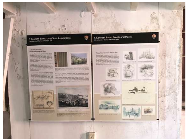
FIGURE 3-86. Plaster damage behind educational posters.
