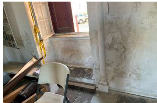
FIGURE 3-51. Plaster damage around Window 1.
