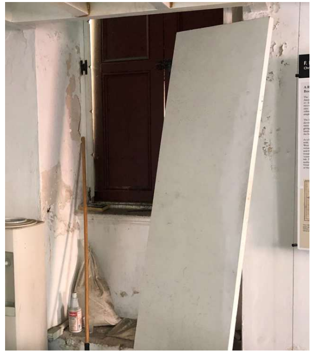
FIGURE 3-85. Plaster damage around Window 11.
