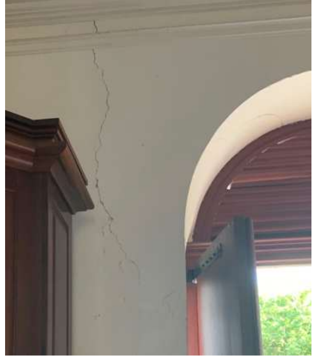
FIGURE 3-77. Large crack next to Door E.
