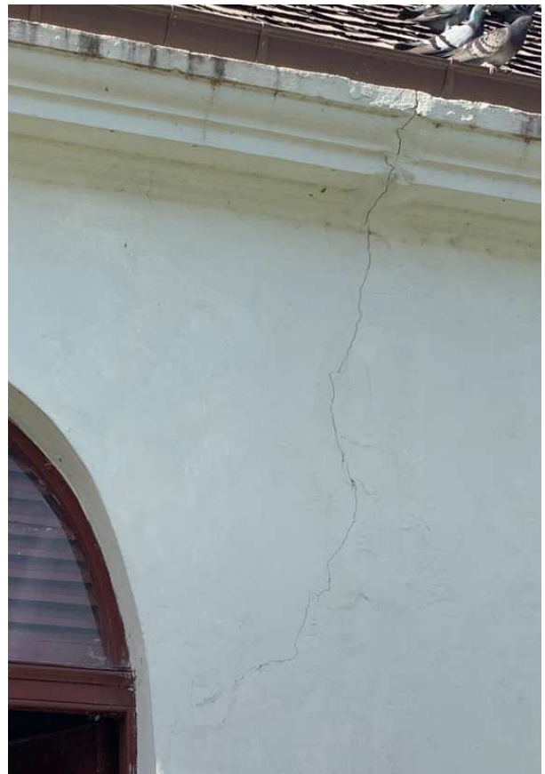
FIGURE 3-24. Large crack near Door E.
