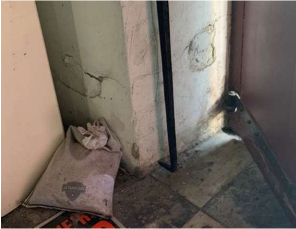
FIGURE 3-74. Cracks to the left of Door D.
