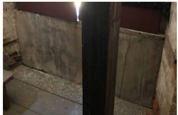
FIGURE 3-108. Cracks under Window 14.
