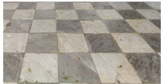
FIGURE 3-94. Cracked and chipped black and white marble tiles.
