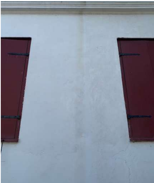
FIGURE 3-17. Staining between Windows 4 and 5.
