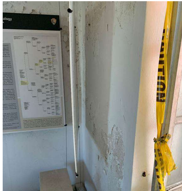
FIGURE 3-49. Plaster failure behind display boards.
