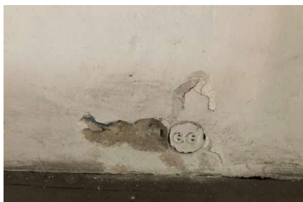
FIGURE 3-89. Plaster damage at left outlet.
