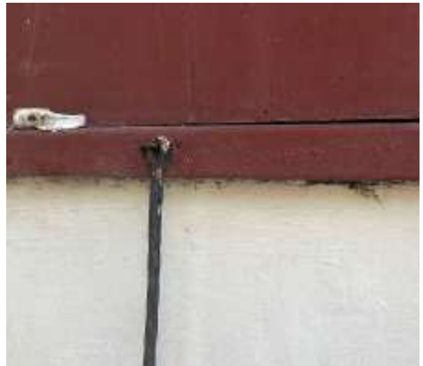
FIGURE 3-172. Gaps in shutters.
