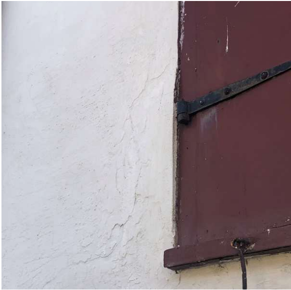
FIGURE 3-13. Bulging in plaster left of Window 6.
