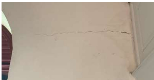
FIGURE 3-80. Crack running from Door E to Window 10.
