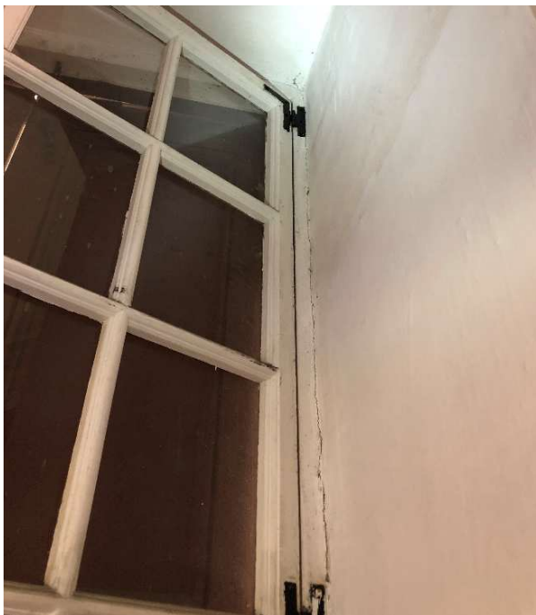
FIGURE 3-92. Crack at edge of Window 12.
