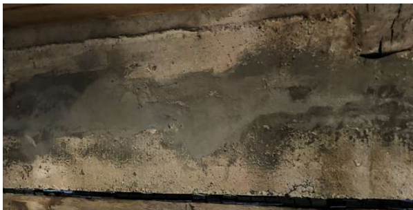
FIGURE 3-124. Concrete patch or repair on northeast wall of third tier.
