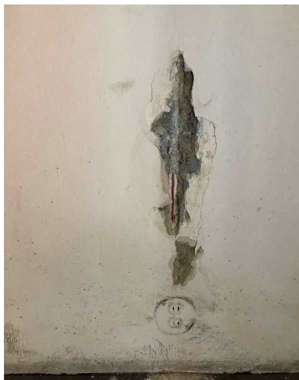
FIGURE 3-91. Plaster damage at right outlet.
