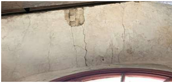
FIGURE 3-119. Series of cracks above Window 14.
