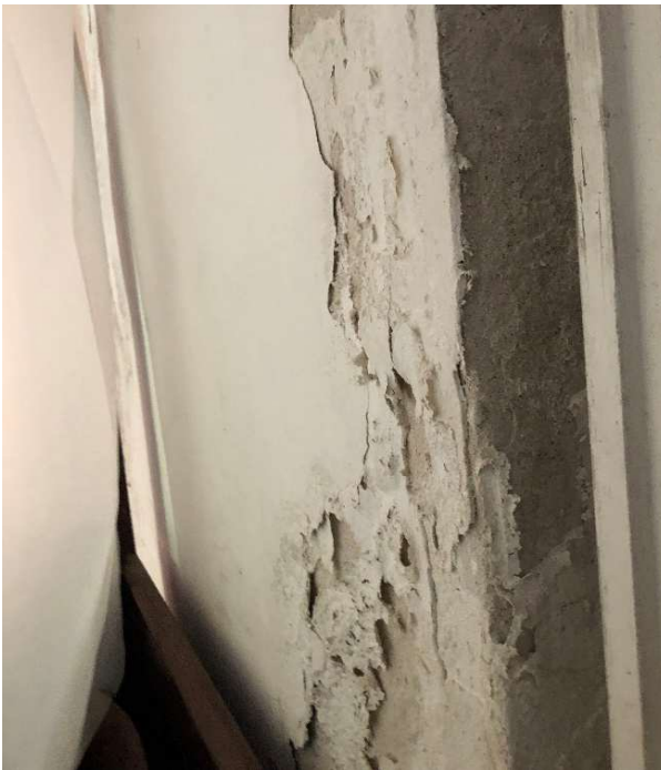
FIGURE 3-53. Plaster damage behind plastic near Window 3.
