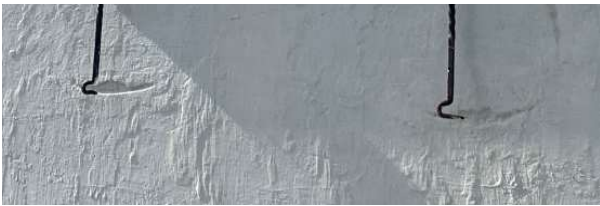
FIGURE 3-22. Grooves cut by shutter hooks.
