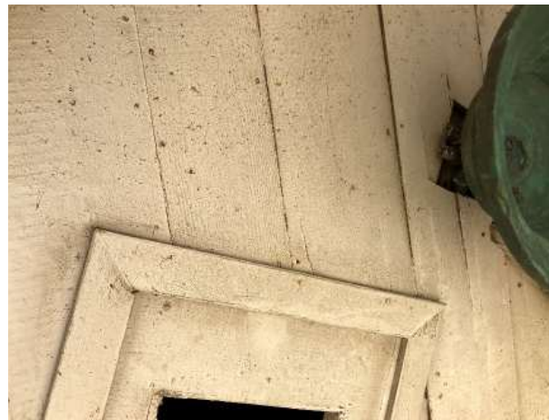
FIGURE 3-144. Slight pitting and cracking of finish layer wood under dome.
