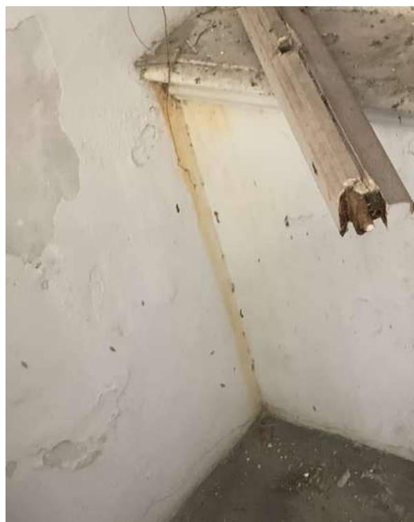
FIGURE 3-83. Rust-colored stain under Window 9.
