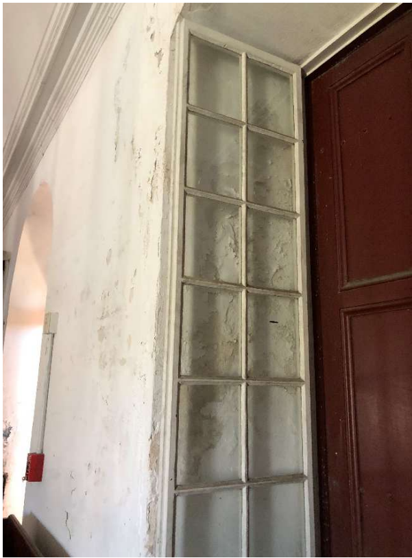
FIGURE 3-56. Plaster damage around Window 4.
