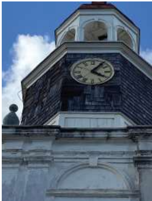
FIGURE 3-162. Missing wood shingles.
