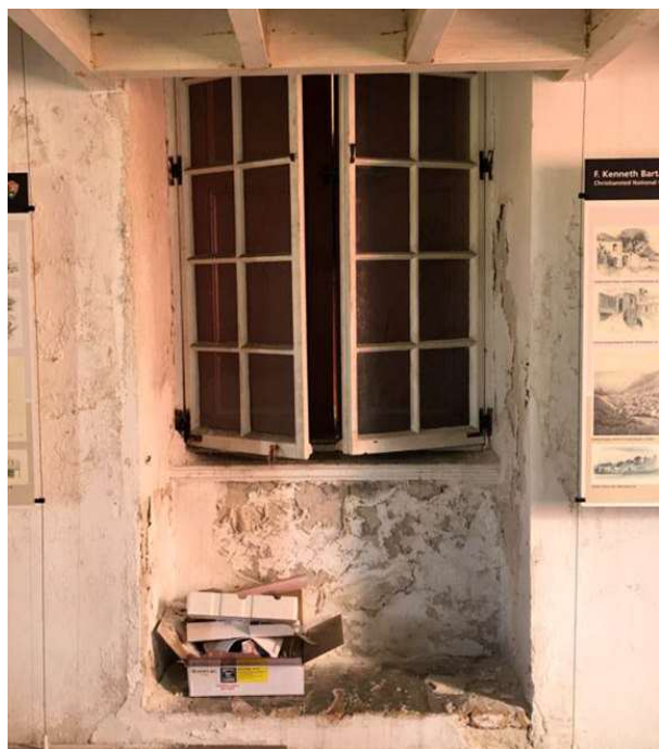
FIGURE 3-87. Plaster damage around Window 12.
