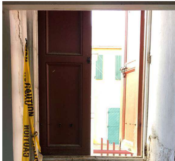
FIGURE 3-67. Missing half of Window 1.
