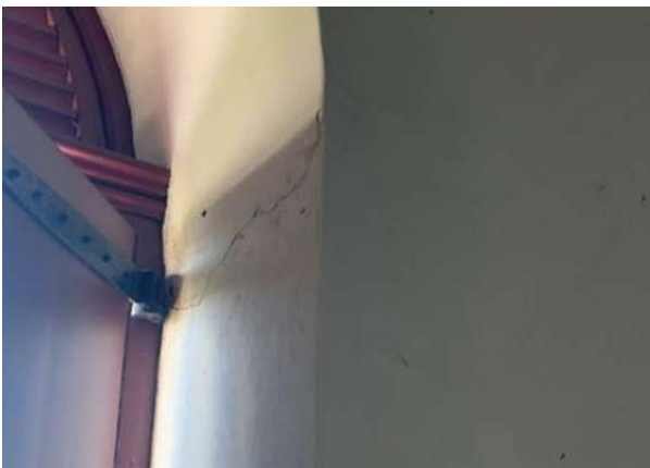
FIGURE 3-76. Crack to the right of Door D.
