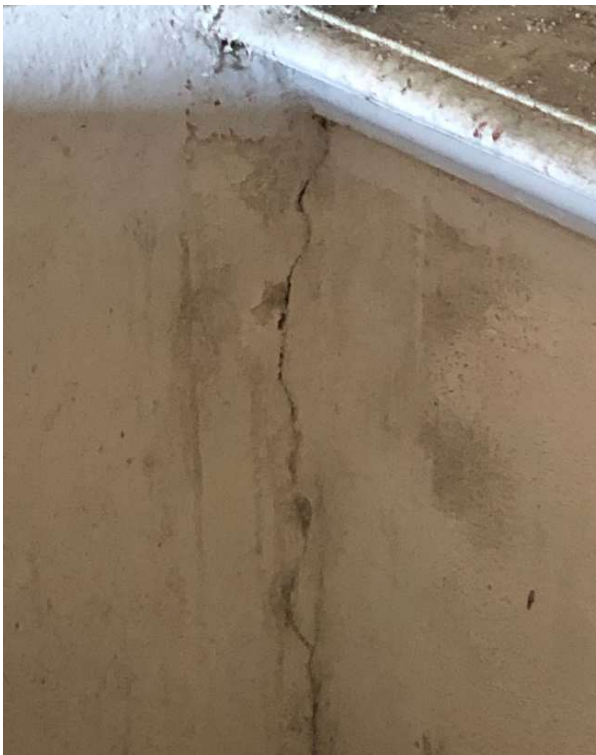
FIGURE 3-62. Crack under Window 4.
