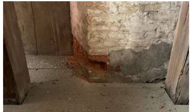
FIGURE 3-107. Brick deterioration right side of second tier, northwest wall..
