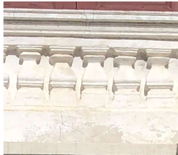
FIGURE 3–43. Cracking in balustrade below Window 15.
