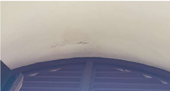
FIGURE 3-75. Crack above Door D.
