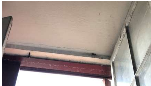
FIGURE 3-59. Crack above Window 2.
