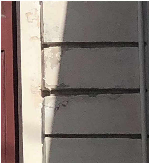
FIGURE 3–41. Plaster damage southwest of Door B.
