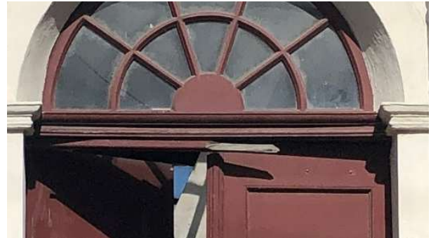
FIGURE 3–42. Broken door frame, Door B.
