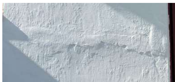
FIGURE 3-28. Patch at lower left side of Door E.
