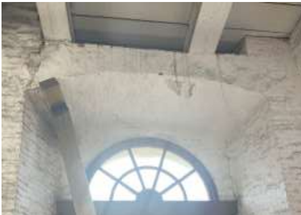
FIGURE 3-165. Vertical cracking above the arched opening at ground level.
