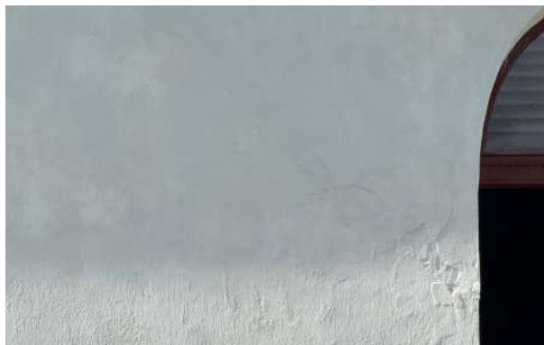
FIGURE 3-27. Patched crack near Door D.
