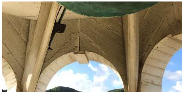
FIGURE 3-145. Slight pitting and cracking of finish layer on back side of cupola arch.
