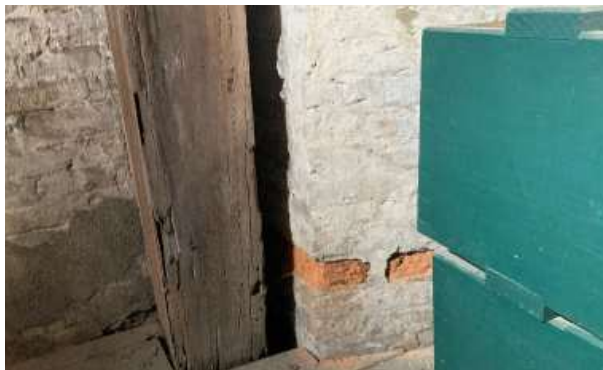
FIGURE 3-111. Brick deterioration left side of second tier, northeast wall.
