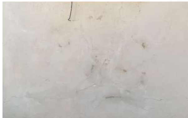
FIGURE 3-11. Cracks under window 6.
