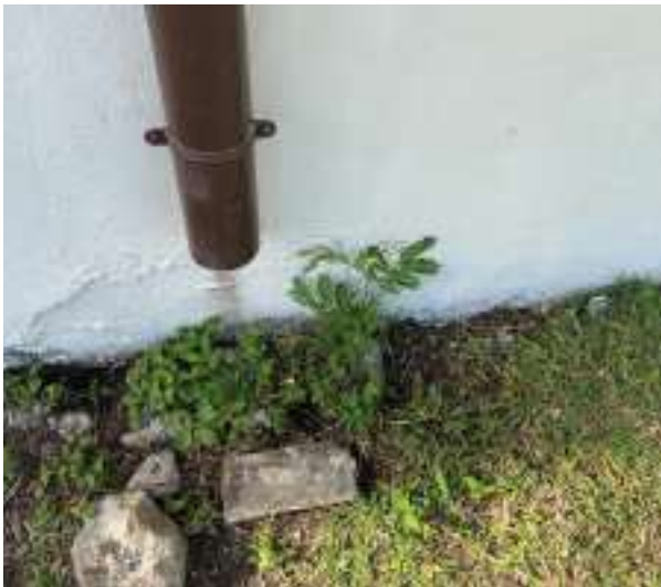
FIGURE 3-171. The downspout is not connected to a drainage line.
