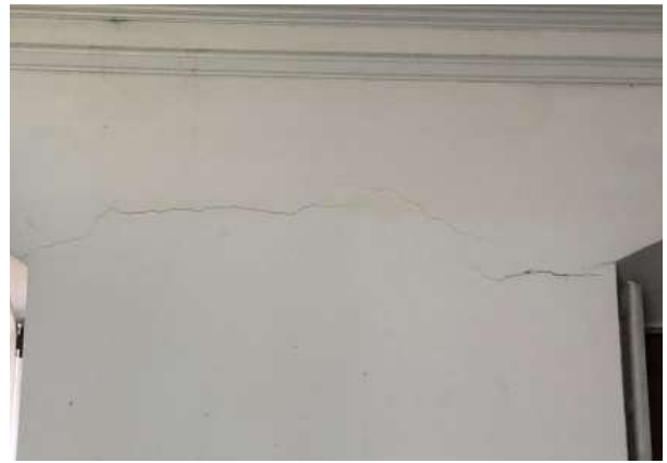
FIGURE 3-63. Cracks between Windows 5 and 6.
