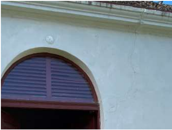
FIGURE 5-9. Example of Settlement Cracking to be Addressed
