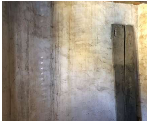
FIGURE 3-113. Water staining on northeast wall of second tier.
