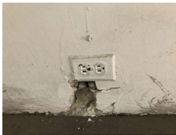
FIGURE 3-90. Plaster damage at middle outlet.
