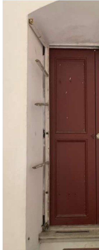
FIGURE 3–72. Broken left half of Window 8.
