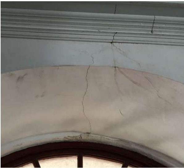
FIGURE 3-61. Crack above Door A.
