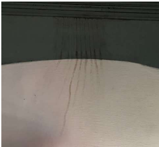
FIGURE 3-65. Stain above Window 2.
