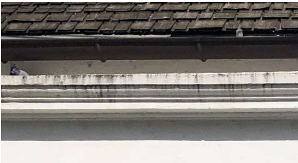
FIGURE 3-32. Staining along the cornice.
