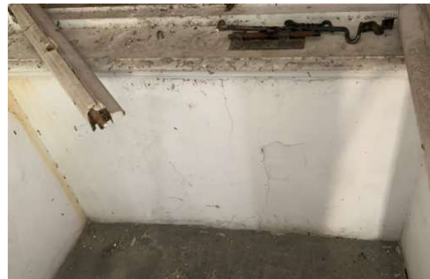
FIGURE 3–73. Cracks under Window 9.
