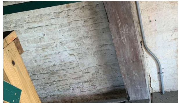
FIGURE 3-125. Crack at right edge of southeast wall of third tier.
