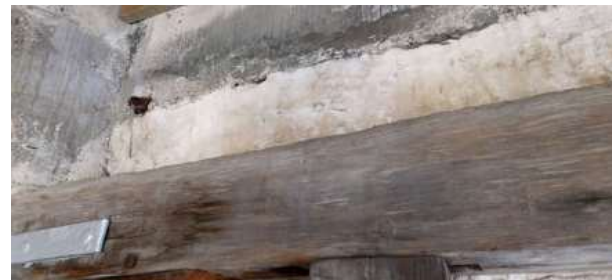
FIGURE 3-126. Series of cracks in the concrete slab above the masonry wall on southeast wall of third tier.
