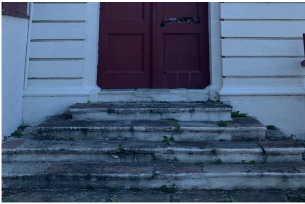
FIGURE 3-35. Steps leading up to Door C with missing section.
