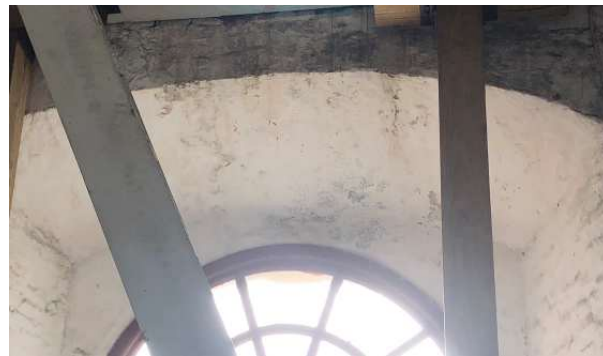
FIGURE 3-105. Crack and paint peeling above Door B.
