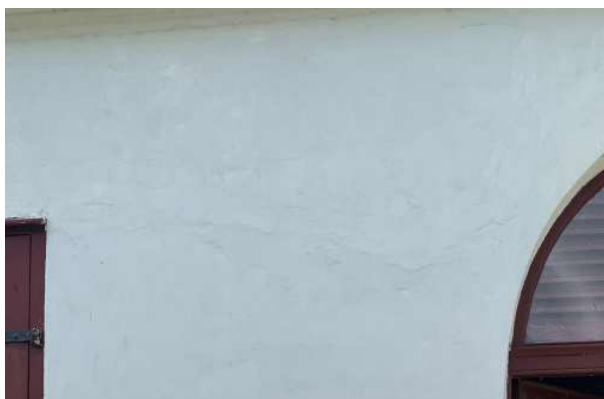
FIGURE 3-25. Patched crack near Door E.
