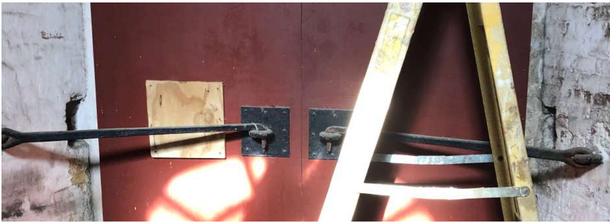
FIGURE 3-102. Empty pockets from past door hardware flank
