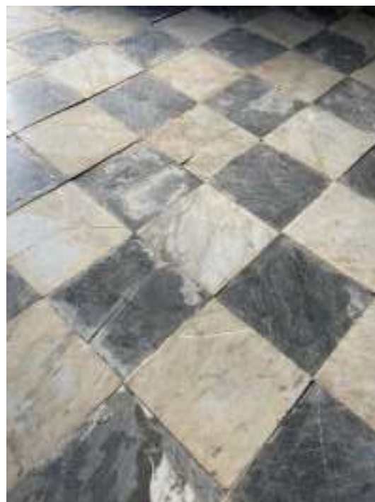
FIGURE 3-152. Cracking observed in tile floor.
