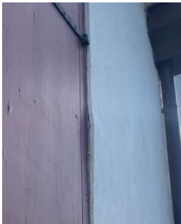
FIGURE 5-4. Bulging at window.
