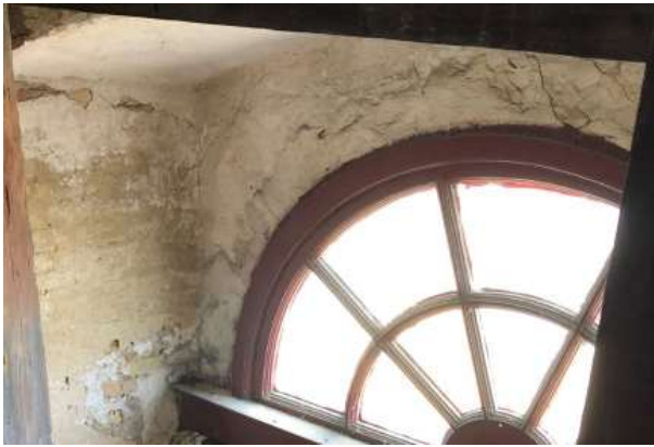
FIGURE 3-120. Series of cracks on either side of the window.
