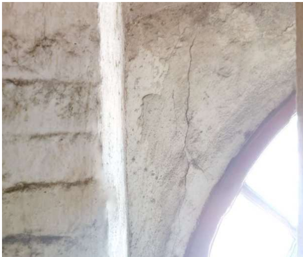
FIGURE 3-129. Crack along left side of Window 15.
