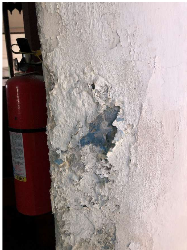
FIGURE 3-66. Blue substance behind plaster.
