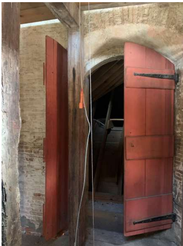
FIGURE 3-115. Door F unable to close left side.
