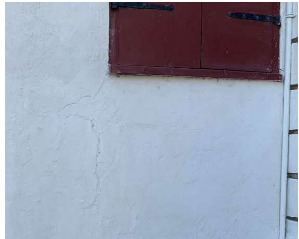
FIGURE 3-15. Cracking under Window 4.
