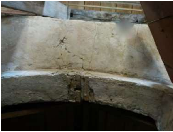
FIGURE 3-114. Crack over the arched opening of Door F.
