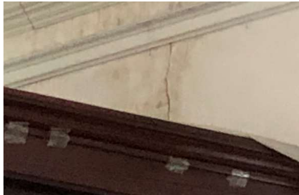
FIGURE 3-60. Crack above Window 3.
