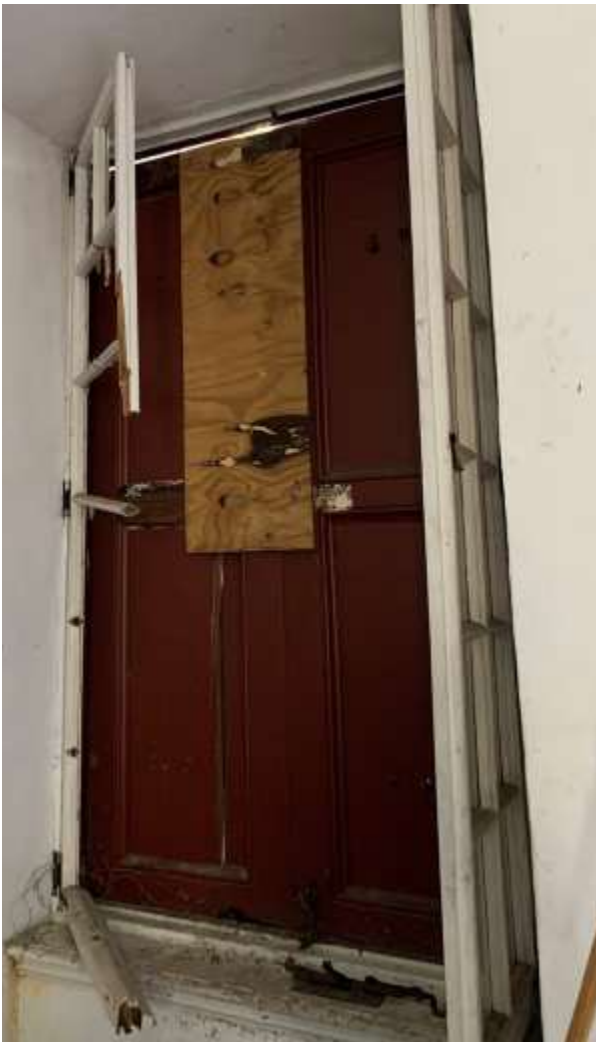
FIGURE 5-5. Example of broken elements at Window 9.
