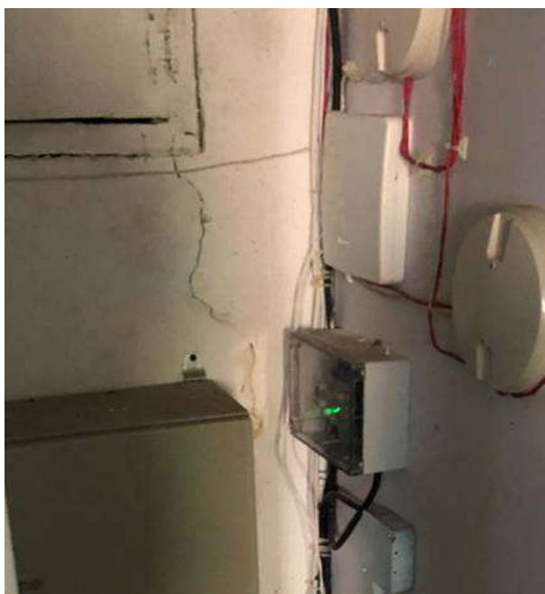
FIGURE 3-81. Crack below access hatch.
