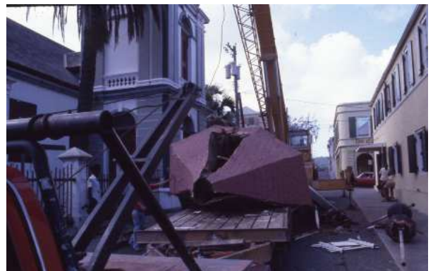
FIGURE 2-39. 1982 photograph of deteriorated cupola loaded on trailer having been removed from Steeple Building. Photo: Christiansted National Historic Site Archives.
