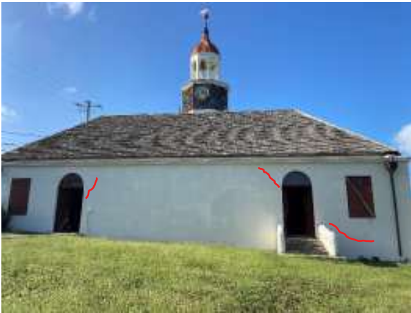
FIGURE 3-154. Observed cracking pattern on the south side. (Figure 3-151).
