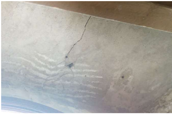
FIGURE 3-128. Crack along arch of Window 15 on southwest wall of third tier.
