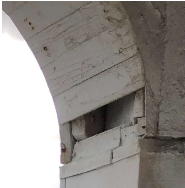
FIGURE 3-143. Rusting of fasteners on cupola
