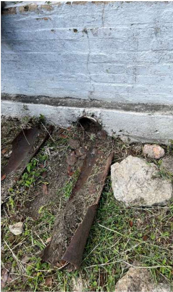
FIGURE 5–8. Broken Hospital Street drain. effects. High pressure washers or other abrasive techniques should not be employed.
