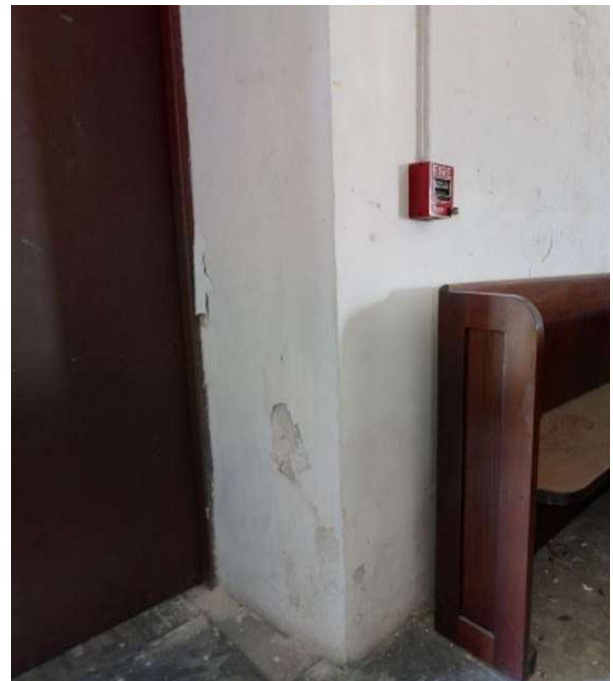
FIGURE 3-55. Plaster damage around Door A's right side.
