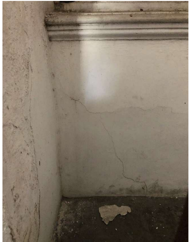
FIGURE 3-64. Cracks under Window 6.
