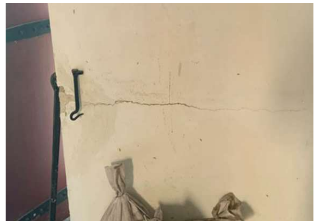
FIGURE 3-79. Cracks to the right of Door E.
