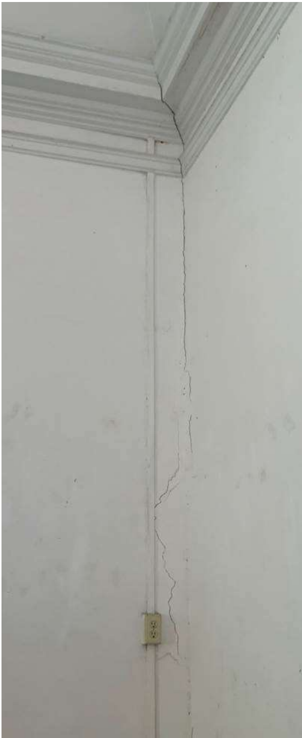
FIGURE 3-69. Crack on right side of northeast wall.
