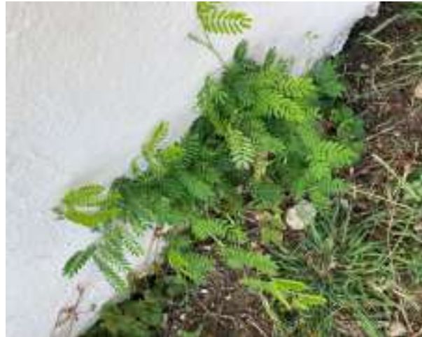
FIGURE 3-151. Root resprouting adjacent to the building
