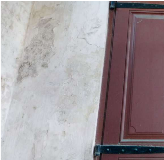
FIGURE 3-104. Plaster failure adjacent to Door A.
