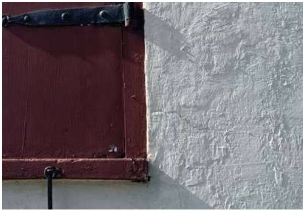
FIGURE 3-21. Small crack near Window 8.
