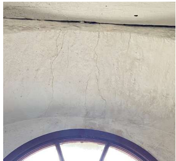
FIGURE 3-164. Vertical cracking above arched openings.
