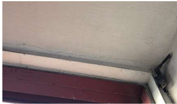
FIGURE 3-58. Crack above Window 1.
