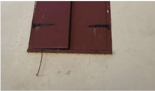
FIGURE 3-12. Cracks around Window 6.
