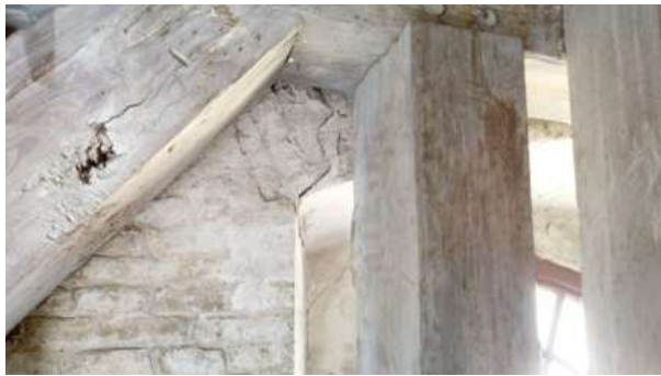
FIGURE 3-121. Crack on left side of arch southwest wall of second tier.
