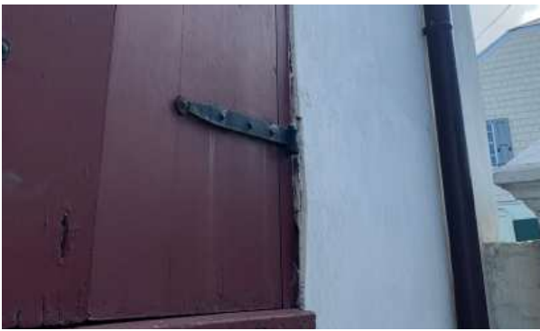
FIGURE 3-3. Bulging on northeast wall.
