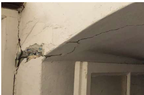
FIGURE 3-82. Crack at Window 10.
