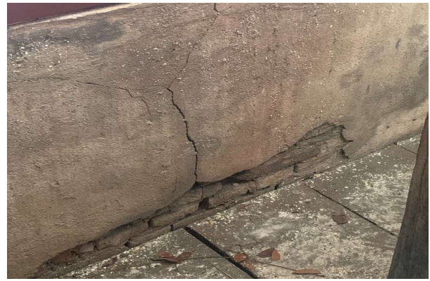
FIGURE 3-116. Series of cracks underneath Window 14.
