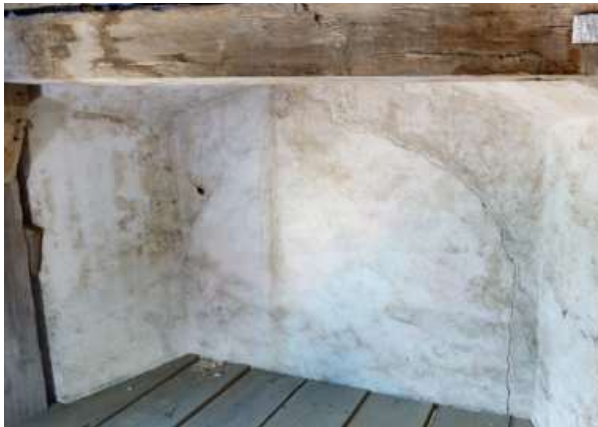
FIGURE 3-123. Series of cracks around infill on northeast wall of third tier.
