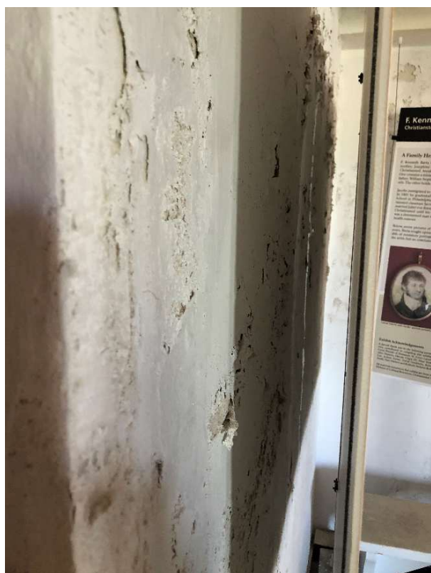
FIGURE 3-88. Plaster damage down wall.
