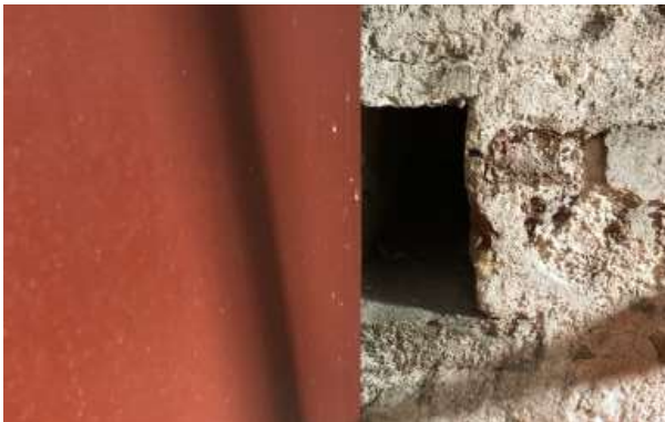
FIGURE 3-103. Empty pockets from past door hardware flank Door C.
