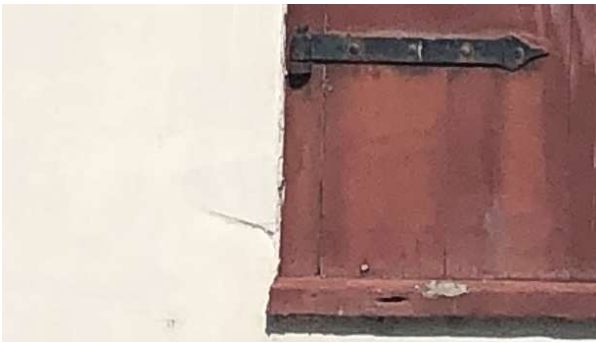
FIGURE 3-31. Crack near the lower left corner of Window 11.
