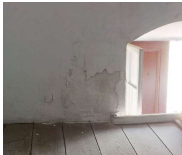
FIGURE 3-50. Plaster damage above mezzanine.
