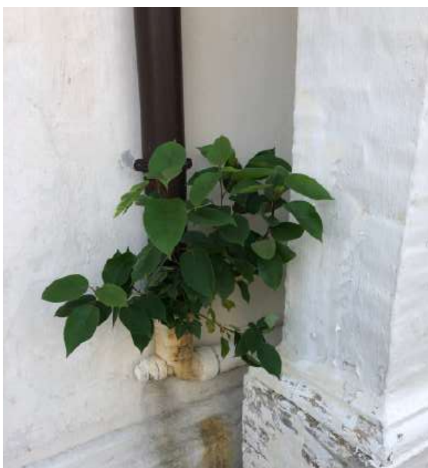
FIGURE 5-7. Plant growing through rain leader.
