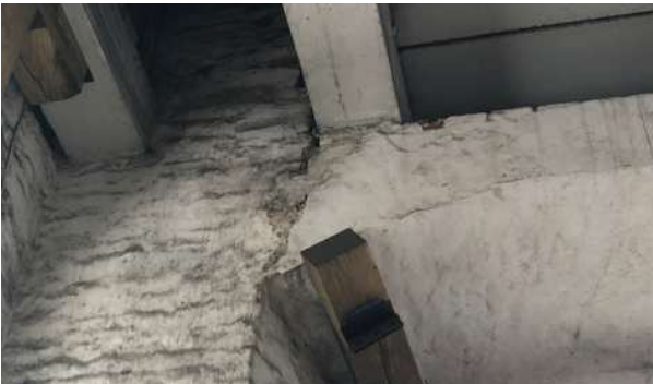
FIGURE 3-100. Large crack above Window 13.
