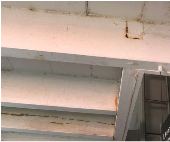
FIGURE 3-98. Rust stains under mezzanine.
