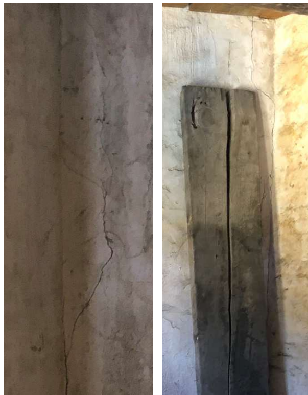
FIGURE 3-112. Cracking on left and right side of wall of second tier, northeast wall.
