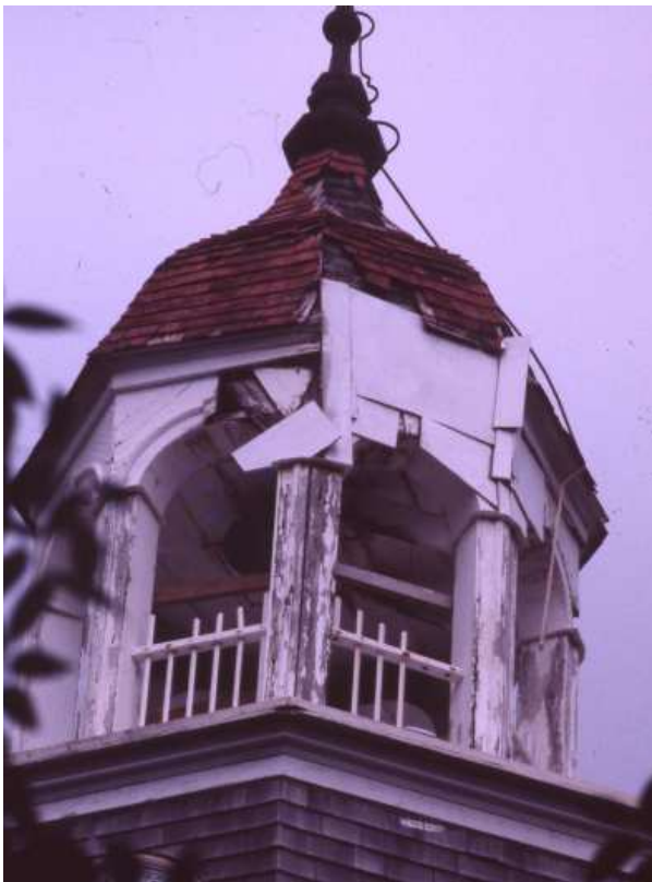
FIGURE 2-37. 1981 photograph of deteriorated cupola on Steeple Building. Photo: Christiansted National Historic Site Archives.
