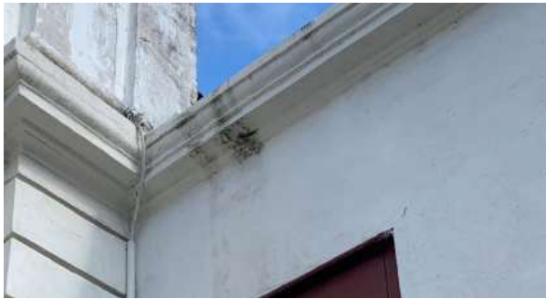
FIGURE 3-4. Staining on northwest wall.
