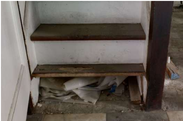
FIGURE 3-99. Broken first step of mezzanine.
