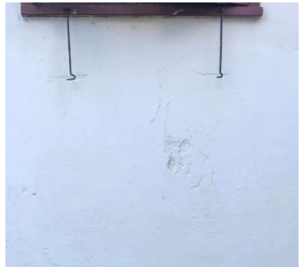
FIGURE 3-16. Bulging in plaster under Window 5.
