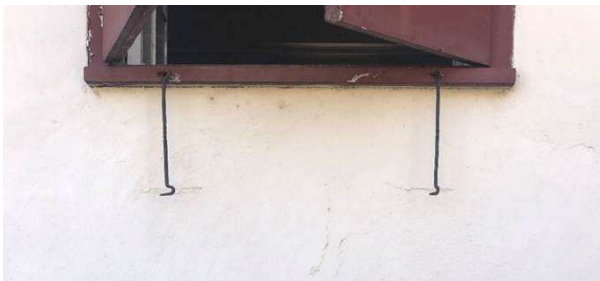
FIGURE 3-19. Grooves cut by shutter hooks.
