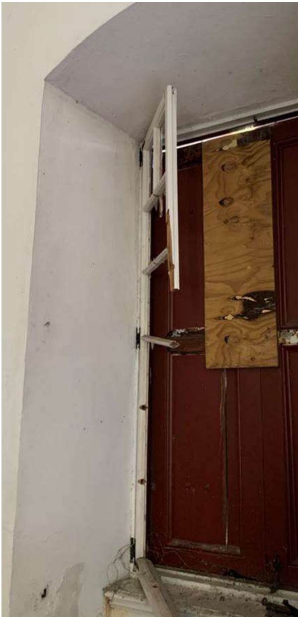
FIGURE 3-84. Broken left half of Window 9.
