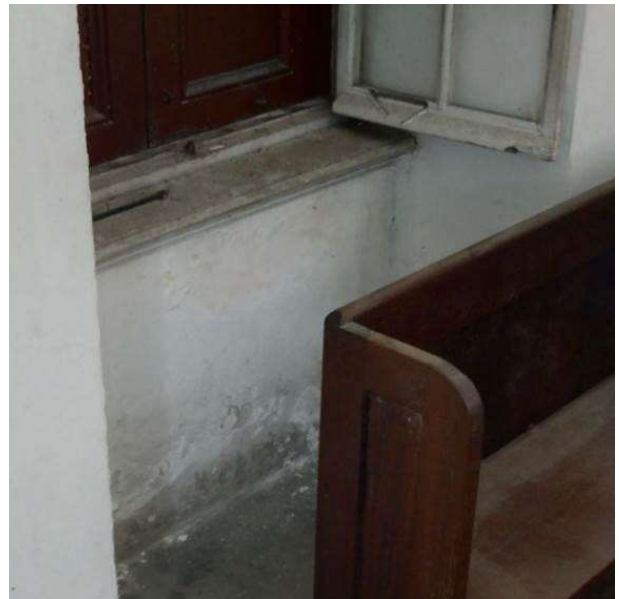
FIGURE 3-70. Plaster damage under Window 8.
