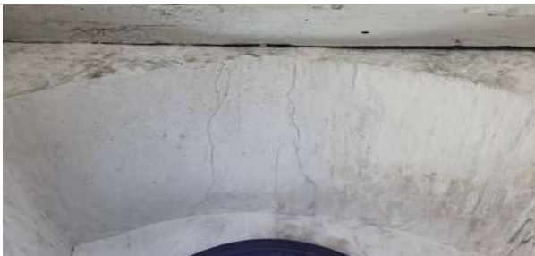
FIGURE 3-101. Cracks above Door C.
