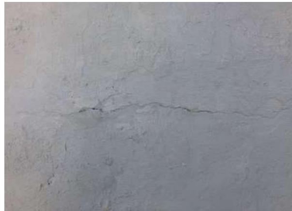
FIGURE 3-20. Crack on northeast façade.
