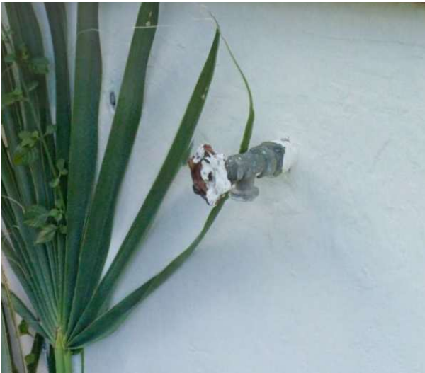
FIGURE 3-23. Penetration near water spigot on southeast façade.
