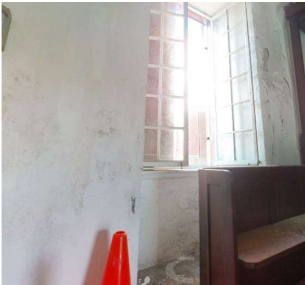
FIGURE 3-52. Plaster damage around Window 2 toward Window 3.
