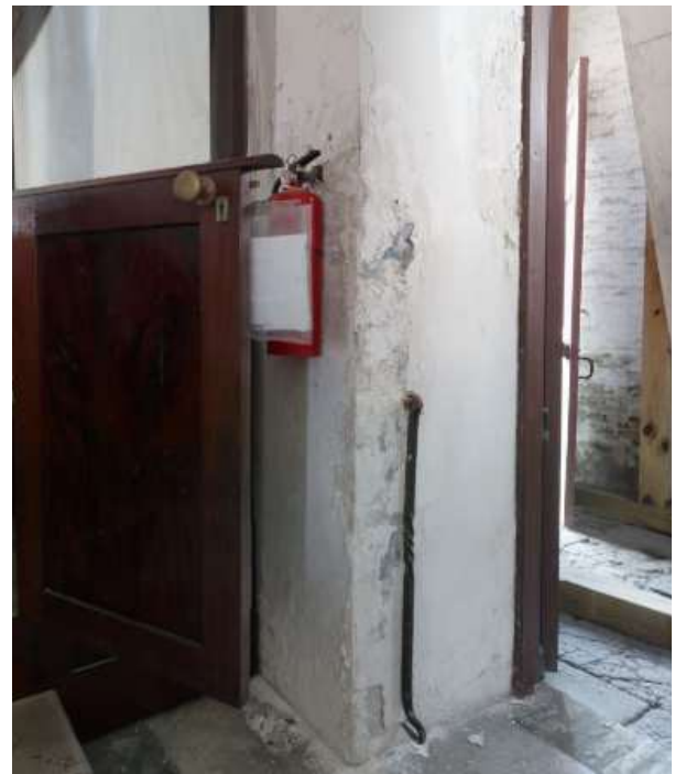
FIGURE 3-54. Plaster damage around Door A's left side.
