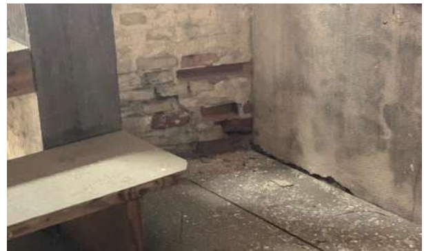
FIGURE 3-106. Brick deterioration left side of second tier, northwest wall.
