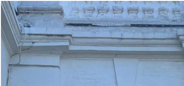
FIGURE 3-36. Cracks in cornice of northeast elevation.
