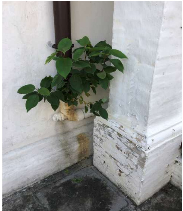
FIGURE 3-6. Plant growing from rain leader.
