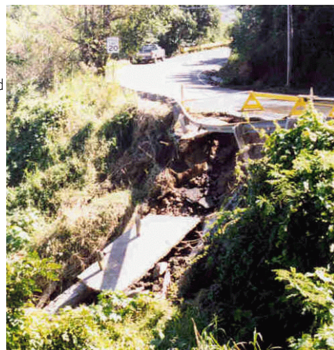
Crown Mountain Road wash-out from clogged culvert after December 2 nd rainstorm.
