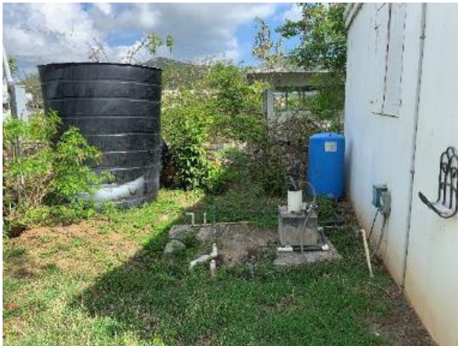
Photograph 4: View of the STEELE well system and associated plumbing which runs across the street to the associated residence shown in Photograph 3 above.
