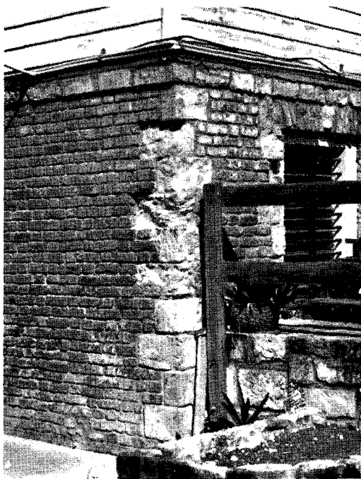
deteriorated stone quoins at Redcliffe Quay
