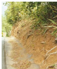
Eroded soil from a denuded roadside clogs Raphune Hill drainage swale.
