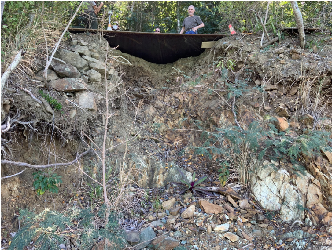
Picture 4. Lyne House Road, Embankment Failure
