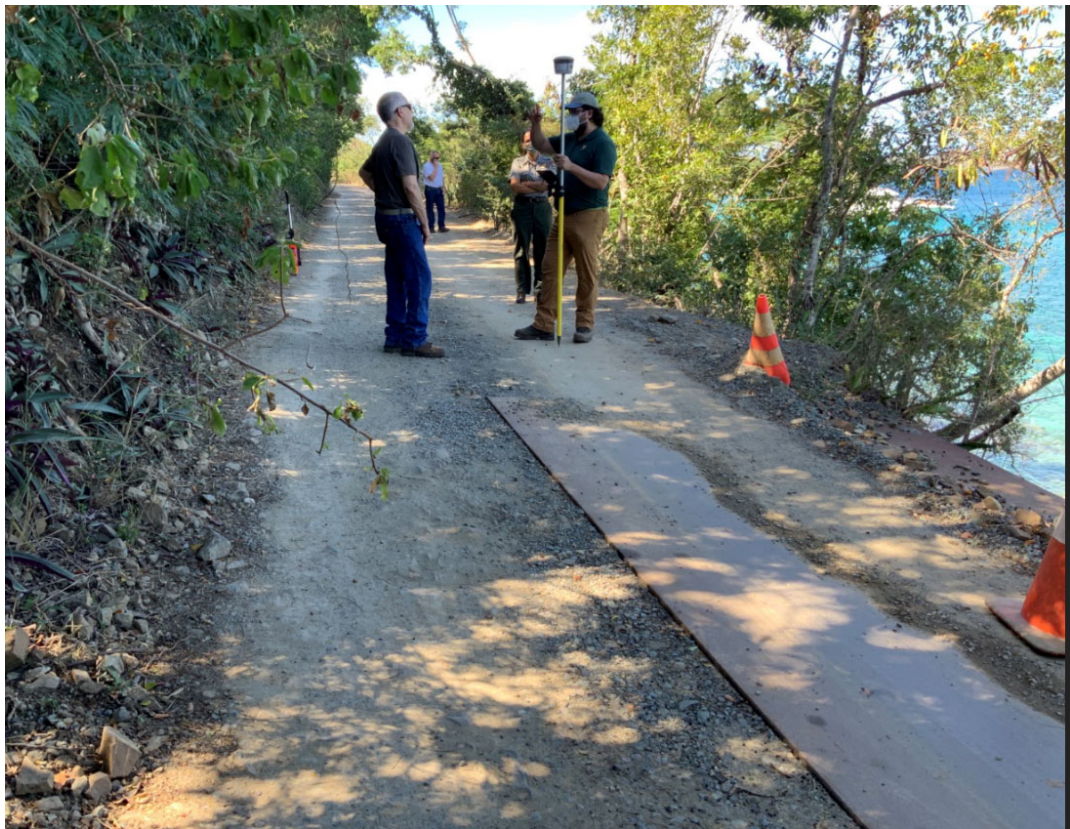
Picture 3. Lyne House Road, Embankment Failure
