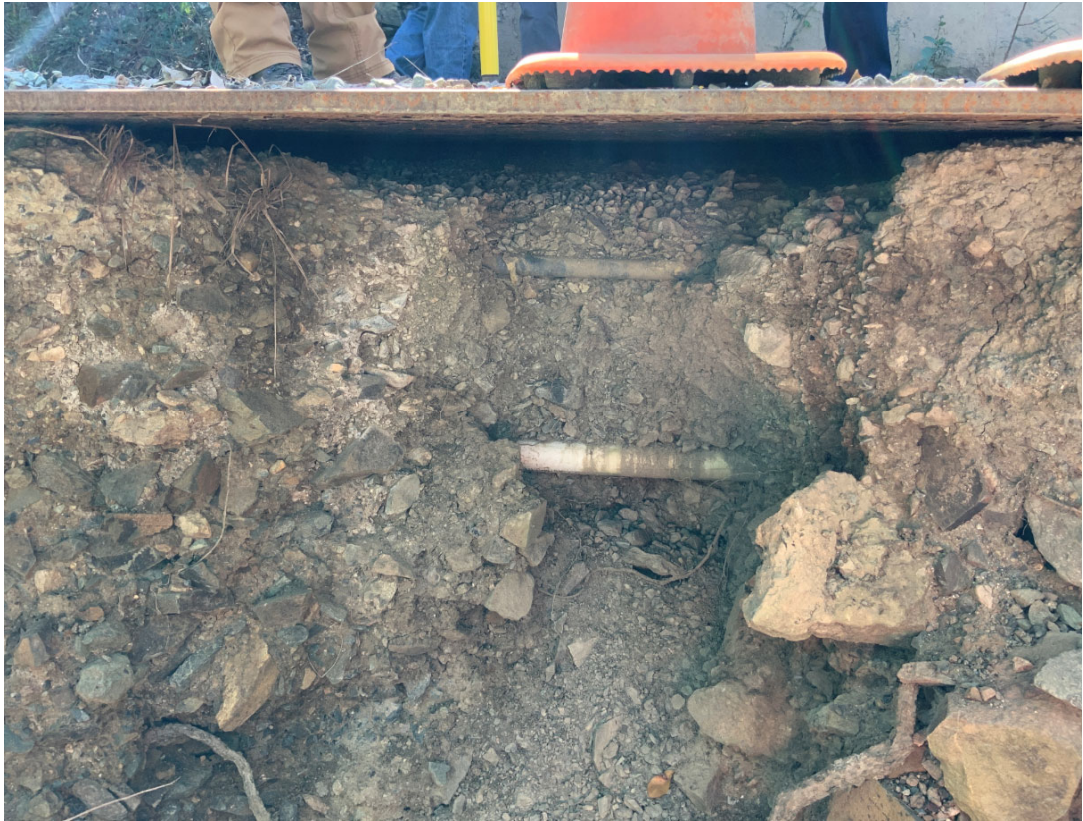
Picture 2. Lyne House Road, Embankment Failure
