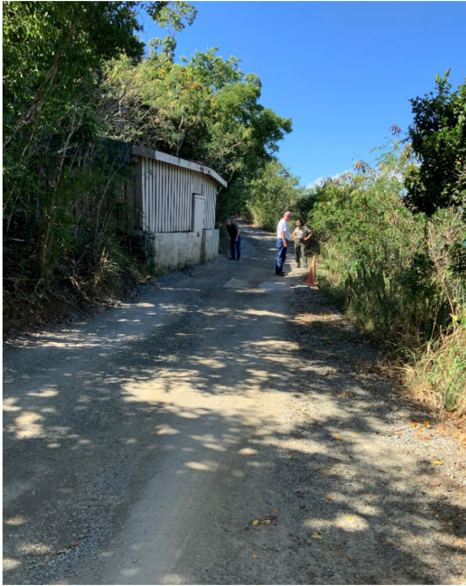
Picture 1. Lyne House Road, Embankment Failure, Reverse Osmosis Facility
