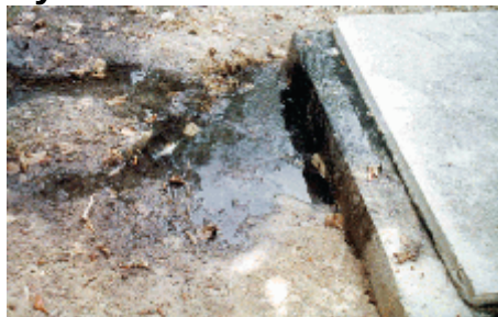
Untreated sewage overflowing from a failed septic system on St. Thomas.
