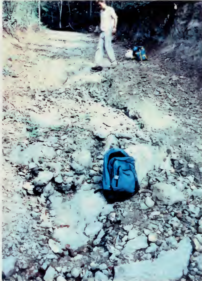
Figure 4.2. Erosion of unpaved road surface.
