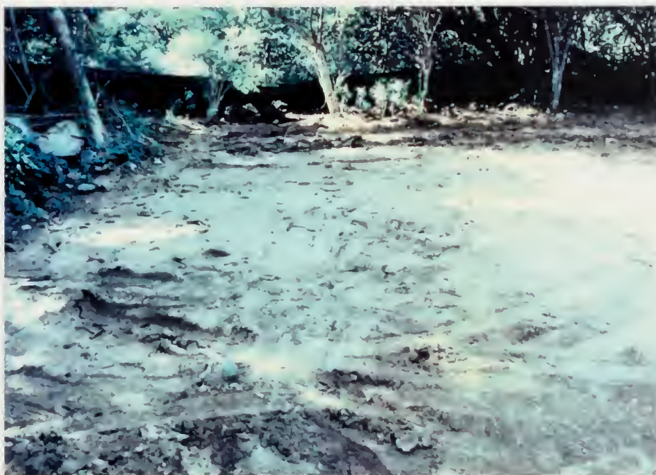
Figure 4.3. Road-derived sediment accumulated behind a sediment fence at Haulover Bay over the first four months following construction.
