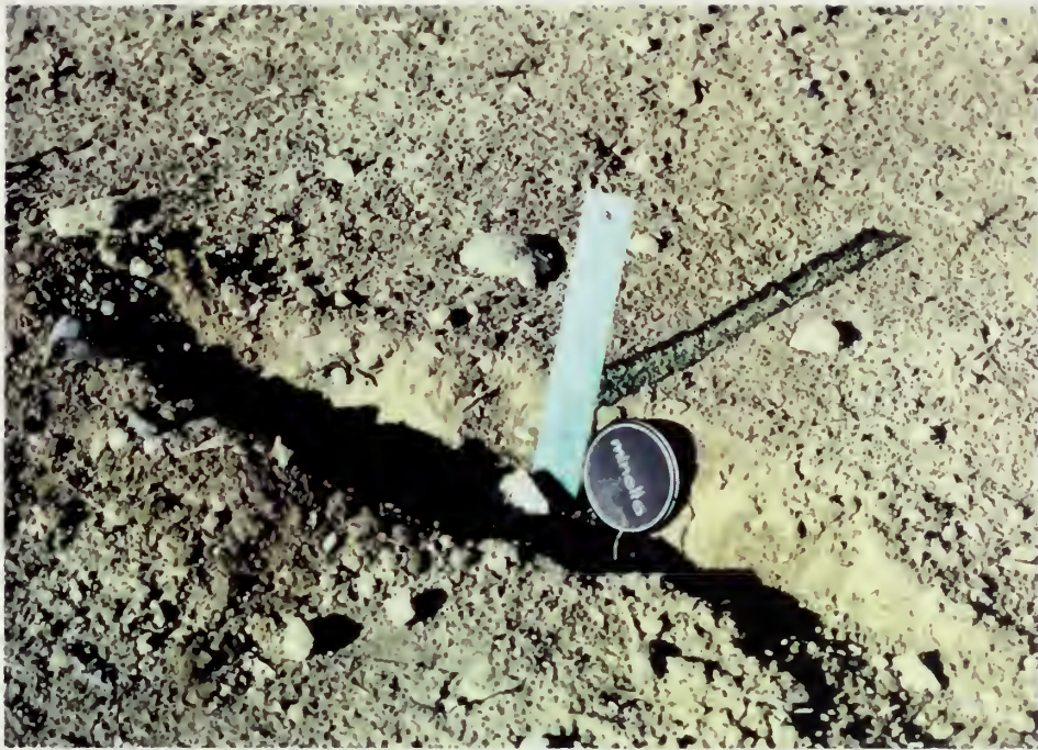
Figure 4.7. Loose, reworked Fish Bay road surface following grading.
