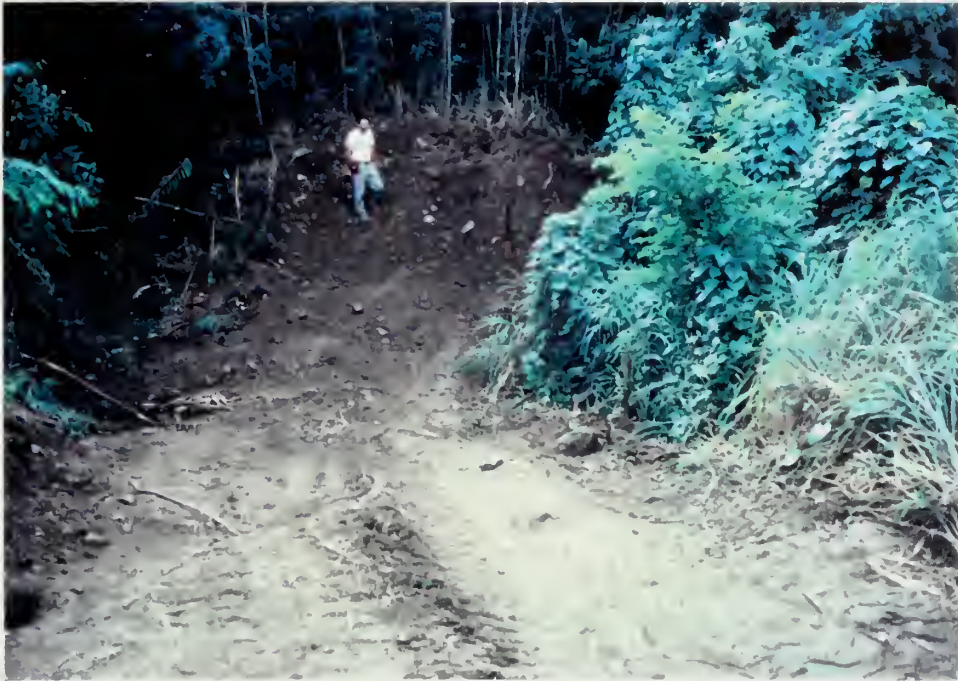
Figure 7.1. Bulldozed swath through Fish Bay Gut, January 1994.
